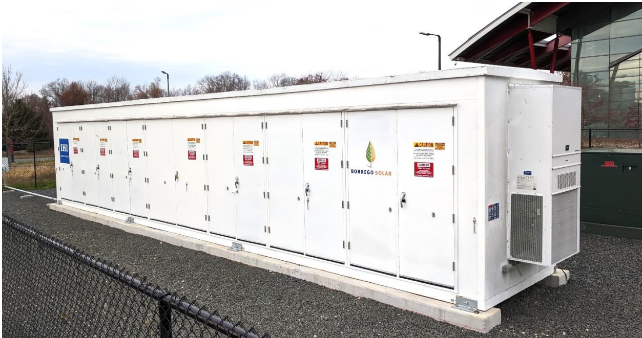
Battery Energy Storage system at UMass Amherst (additional data )
